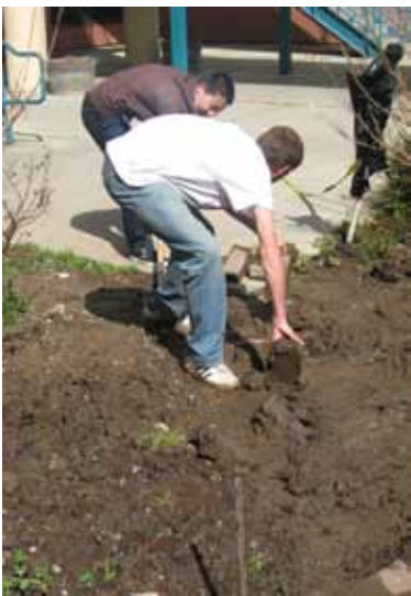
Photo by Kaylee Miu Seniors Ben Rich and Paul Sun help build the new pathway outside the Eggers building.
